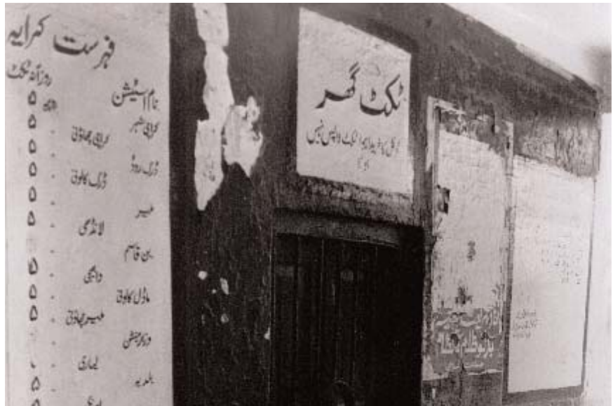
Multitude of structural shortcomings at the rail ticket office.
