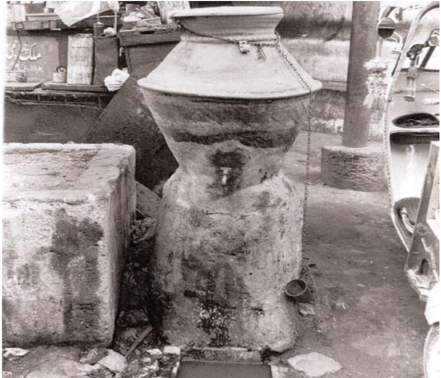
Too close for comfort—public drinking water in close proximity to sewage water.
